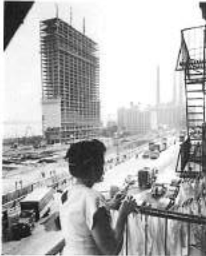
A woman knits as she looks at the steel structure of the United Nations Secretariat Building from a fire escape in New York.
